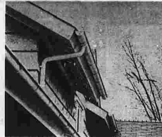
PEELING PAINT under eaves can be corrected by sanding and washing before repainting, say Sherwin-Williams painting experts. Recommended solutions for house paint failures are in a free booklet available at more than 1,500 Sherwin-Williams Decorating Centers nationwide.
